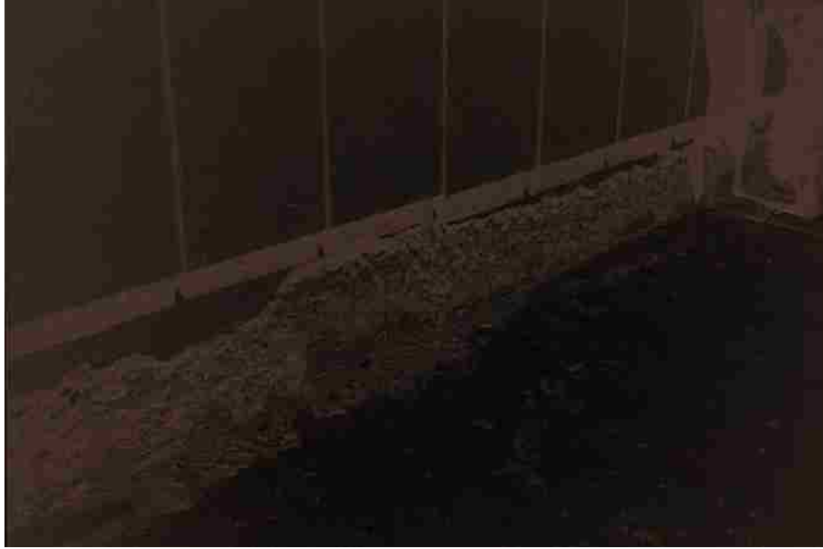
Figure 1-9: Scaling of Concrete Foundation Slab due to Physical Sulfate Attack (Haynes et al. 1996)
