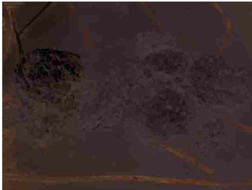
Figure 1-5: Example of Severe TSA Damage in Lab Samples (Rahman & Bassuoni 2014)
