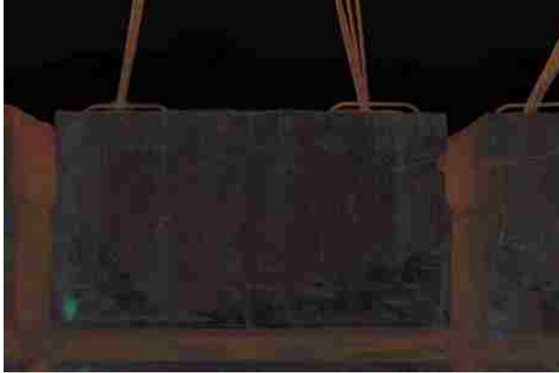
Figure 1-6: Effect of Combined ASR and DEF on Precast Beam (Skalny et al. 2002)
